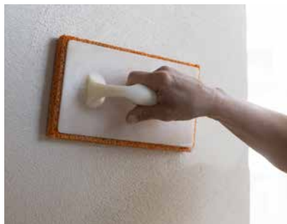
Start first felting pass when plaster has dried from wet to moist.
